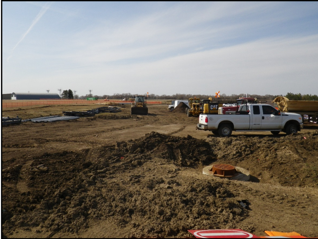
Figure 23: Disturbed portion of APE to the northwest of airport terminal, view to the northwest.
