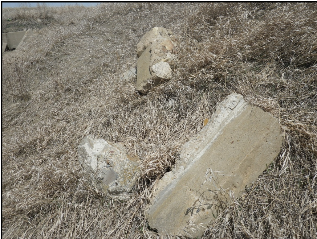
Figure 4: Close-up of concrete pieces within the newly recorded portion of site 39SK988.
